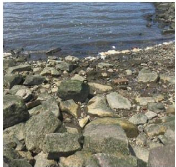
Figure B: View of the seine beach next to the bulkhead, shows boulders and cobbles displaced by waves (2020)
