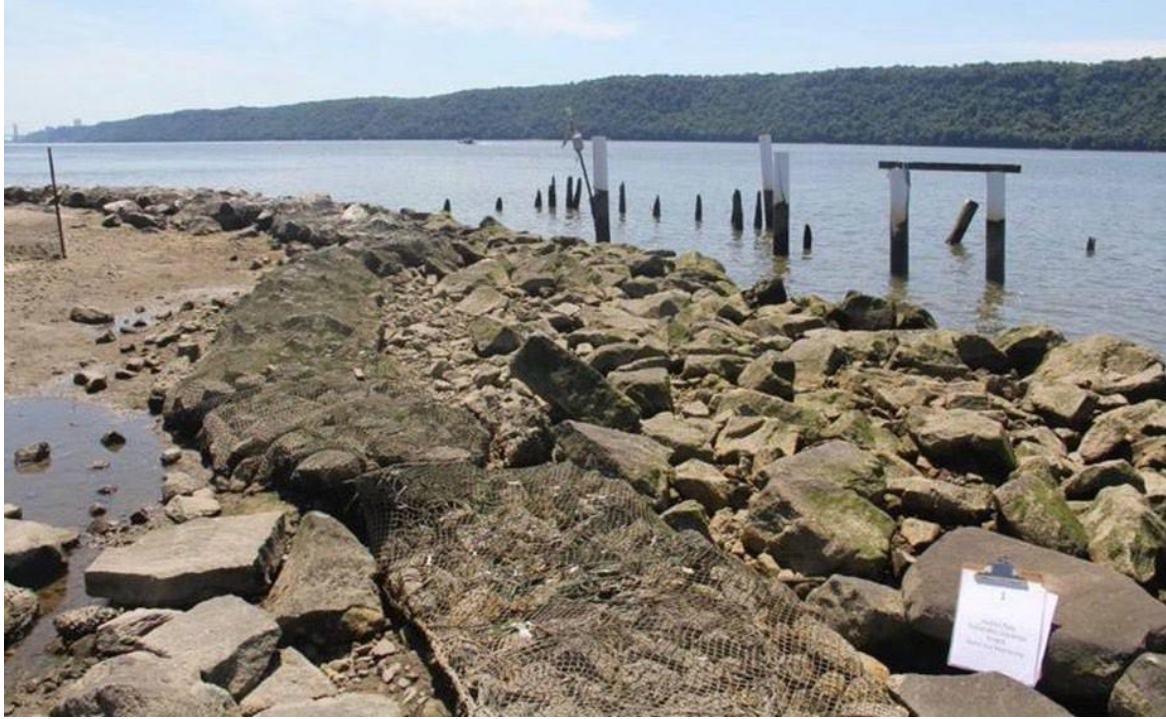
Figure E. View looking southwest at the rock sill in September, 2020. Rock sill continues to provide a protected tidal pool environment. While the netting that encloses the top layer of rip-rap remains intact, some boulders and cobbles without netting have been displaced on the sill.
